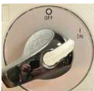
Master Power Switch
